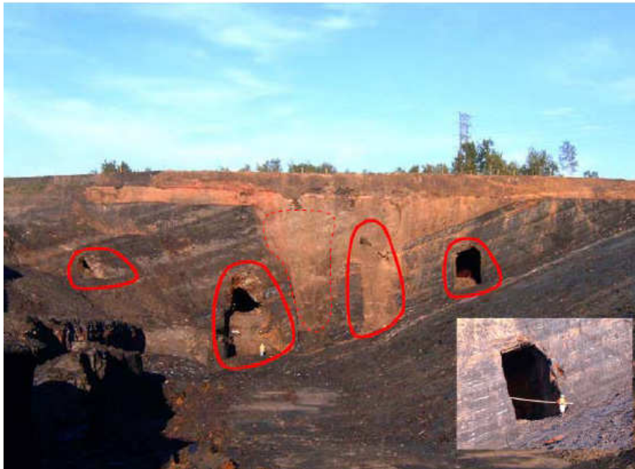
Figure 7.1: Old mine tunnels (red lines) and collapse (dashed lines) in the east boundary of the Stellarton pit (from Xu 2008).
