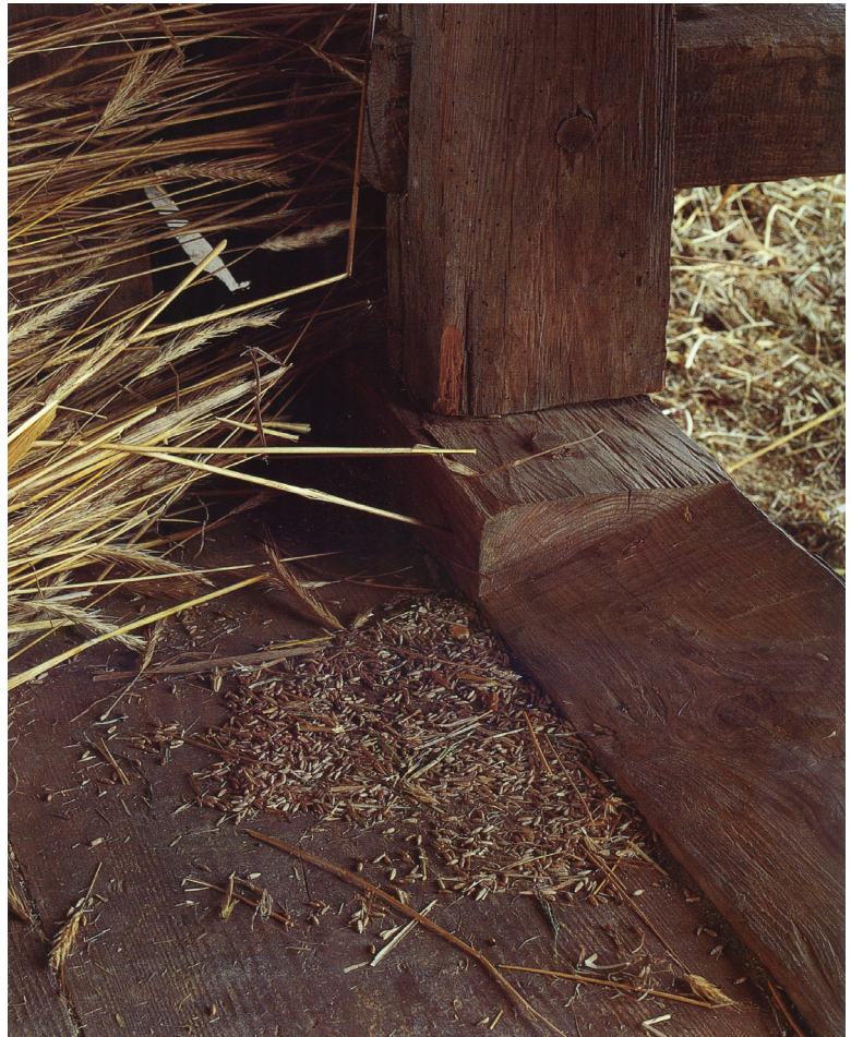
A bevel cut out of the sill of door opening of a wood granary ensures any grain that falls on the sill automatically slides back into the granary floor as opposed to spilling onto the ground outside, Appalachian region. Photograph by Paul Rocheleau, Barn: The Art of a Working Building .
