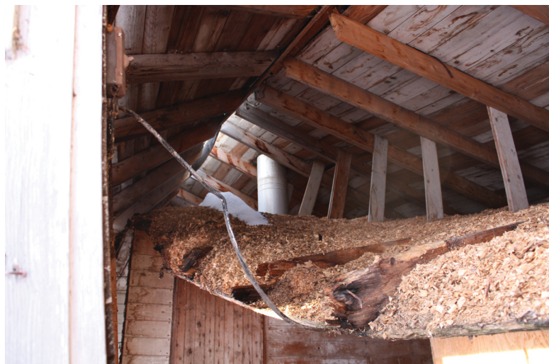
Chicken coop: wood chips as roof insulation.
