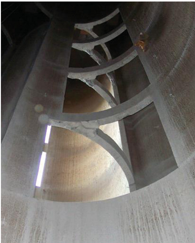
Figure 22: A view up the cuts in the silo for stairs. (Globe Mills 2008)
