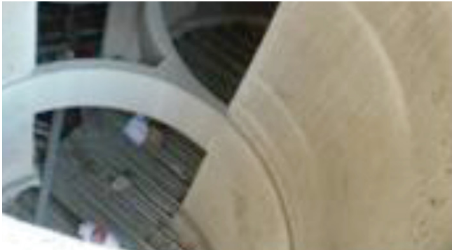
Figure 21: A view down the cuts in the silo for stairs. (Globe Mills 2008)
