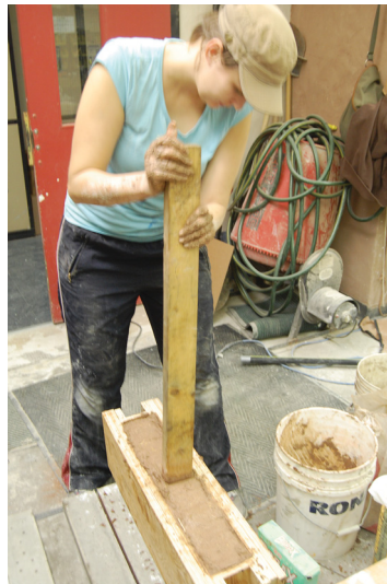
The earth layers were hand tamped and compacted around the threaded rod supports. The earth mixing and tamping were labour intensive.
