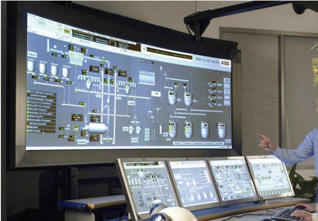
Figure 16. Existing control room operator's screen display.
