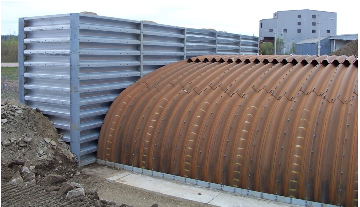
Figure 4-1 – Unburied structure with “Bolt-A-Bin” end treatment
