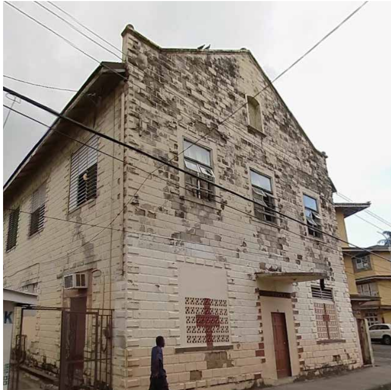
Figure 9. One of many dilapidated buildings on the east side of downtown POS (Google Maps 2024)
