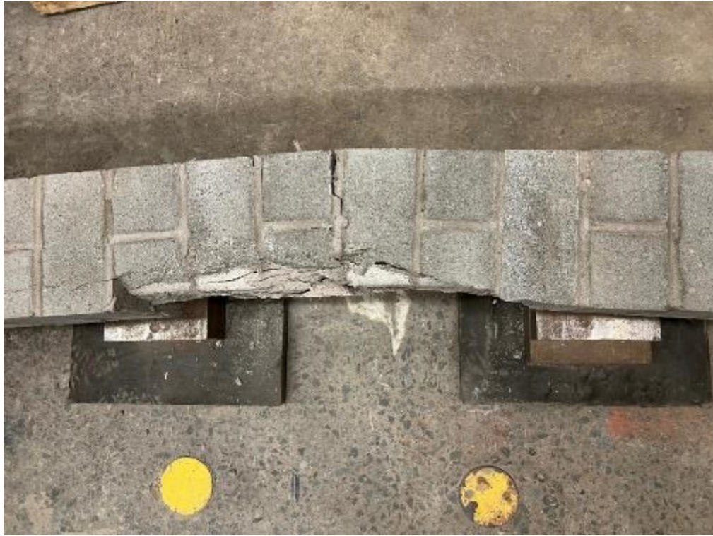
Figure 4.6. Tensile mortar joint crack openings and longitudinal compressive cracks in masonry in specimen MC.
