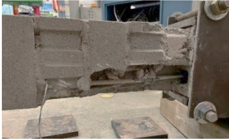
Figure 4.11. Closeup of pre-mature failed area for specimen MS.
