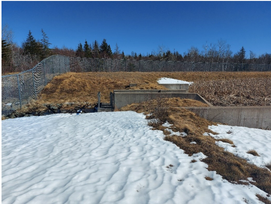
Figure A.16 Outlet structure of constructed wetland for System 1.
