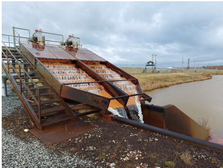
Figure A.1 Aeration cascade with high flow at settling pond inlet for System 1.
