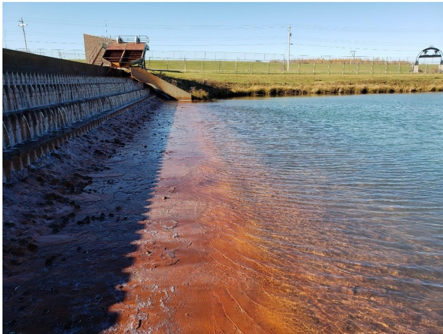
Figure A.4 Inlet distribution structure after aeration cascade with low flow at settling pond inlet for System 1.
