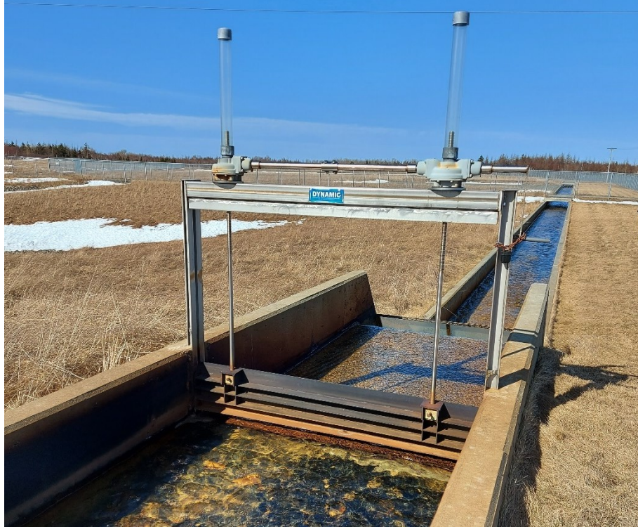
Figure A.13 Sluice gate in channel between settling ponds and constructed wetland for System 2.
