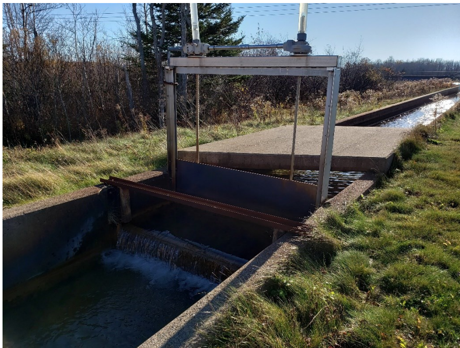
Figure A.12 Sluice gate in channel between settling pond and constructed wetland for System 1.
