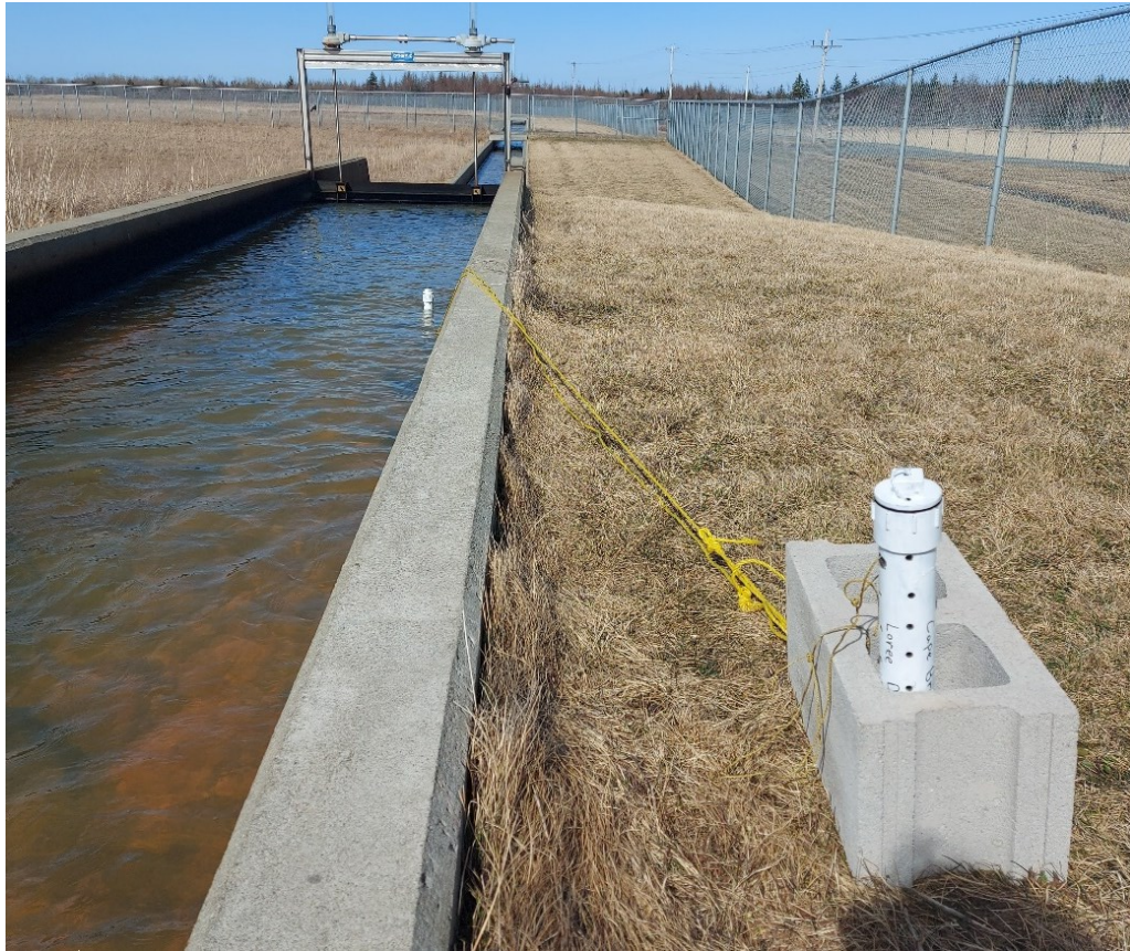
Figure 3.6 HOBO pressure transducers with high flow in channel between settling ponds and constructed wetland for System 2.
