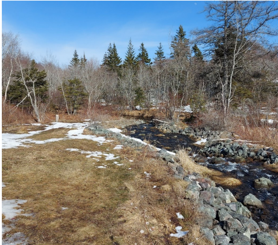
Figure A.18 Combined discharge channel for System 1 and System 2 flowing to Cadegan Brook.
