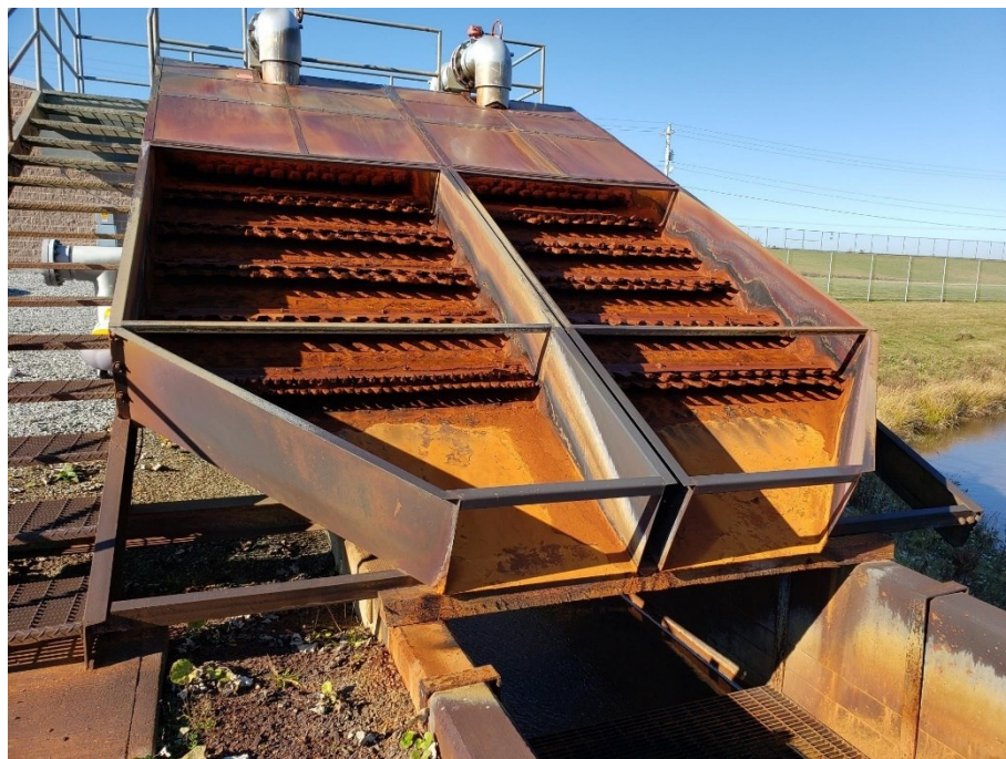
Figure A.2 Aeration cascade with no flow at settling pond inlet for System 1.
