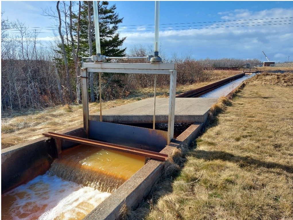
Figure 3.7 Sluice gate in channel between settling pond and constructed wetland for System 1.
