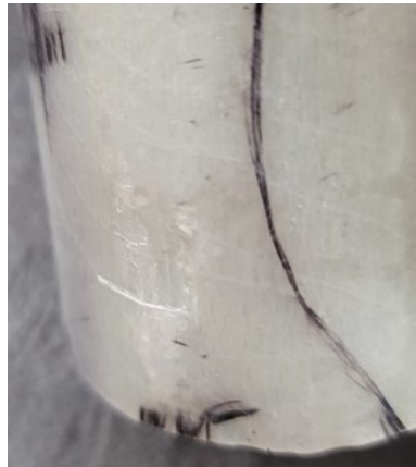
Figure 5-6 Local surface wrinkle caused by the overheated shrink tape.
