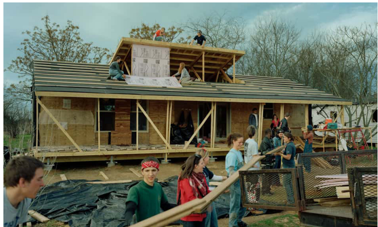
Fig. 10 Students at Rural Studio work together to build Rose Lee’s house (Freear et al. 2014, 70).
