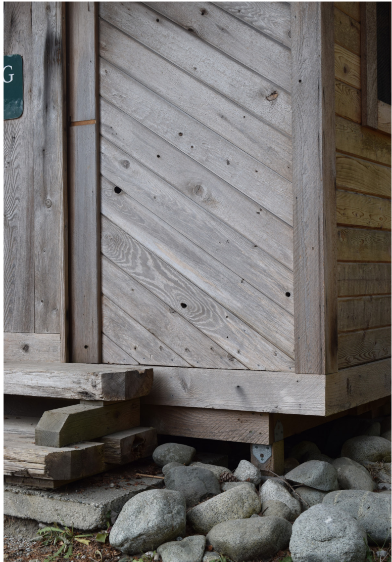
Fig. 29 A detail of siding and foundations of a recycling shed for a retreat on Cortes Island.
