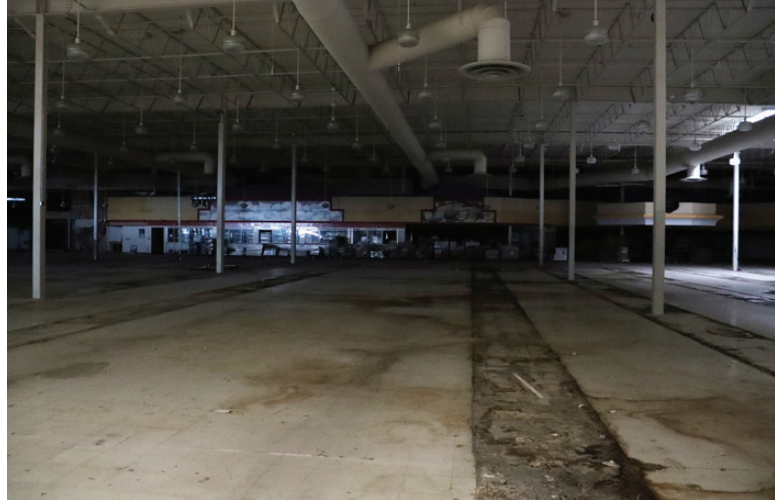
Interior image of existing building on proposed site, demonstrating current conditions of building.
