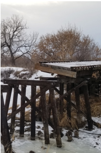
Figure 25: Old rail cart line between Alberta Brick and Tile and Medalta Potteries sites.
