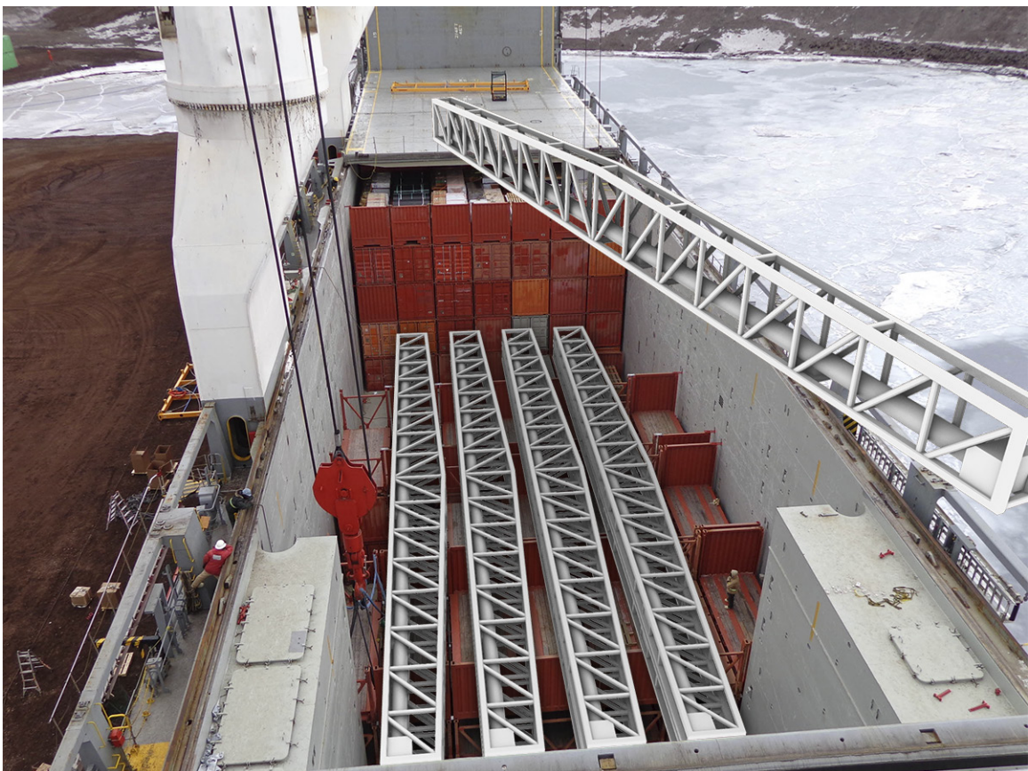
Figure 27: Unloading large prefabricated trusses for factory assembly area. Original photograph by J.F.Alexander (Burford 2013)
