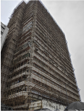
Bamboo scaffolding in various scales around building facades which are commonly found throughout Hong Kong.
