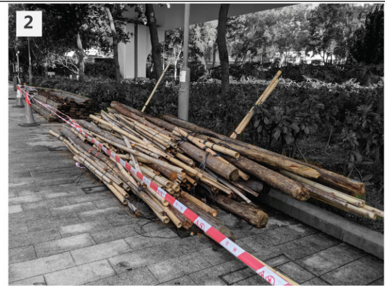
2 Bamboo and wood members stored on sidewalks or placed near the sites.
