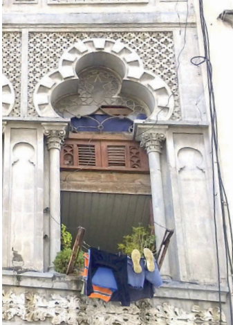
Conditions in the Palacio de las Ursulinas : self-built vertical subdivisions ( barbacoas ) can be seen facing the street, adding load to the deteriorating structure below.
