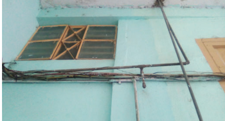
Ad hoc installations of gas and electrical conduits in the building (Pérez et al. 2019).
