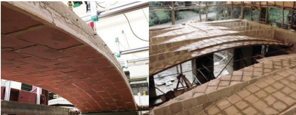
Left: research into the use of Catalan or timber vaults as integrated formwork for reinforced concrete, acting as a composite structure (López López et al. 2019, 240). Right: shallow timber vaults with collar ties in the Sustainable Urban Dwelling Unit project (Block, Van Mele, and Rippmann 2015).
