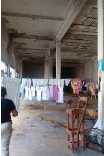
The common utility area on the second floor of Ursulinas (Pérez et al. 2019).
