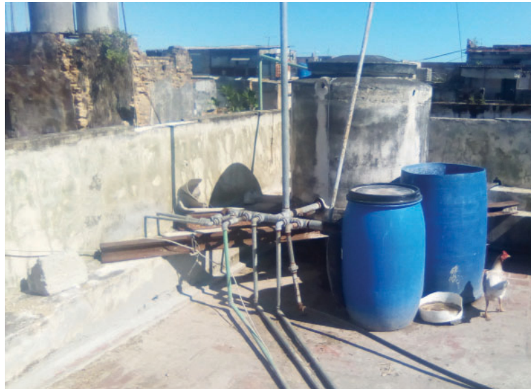
Rooftop containers for domestic water supply (Pérez et al. 2019)
