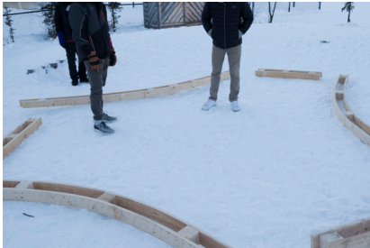
Laying out the footprint, only to decide that the connectors should be a bit larger.
