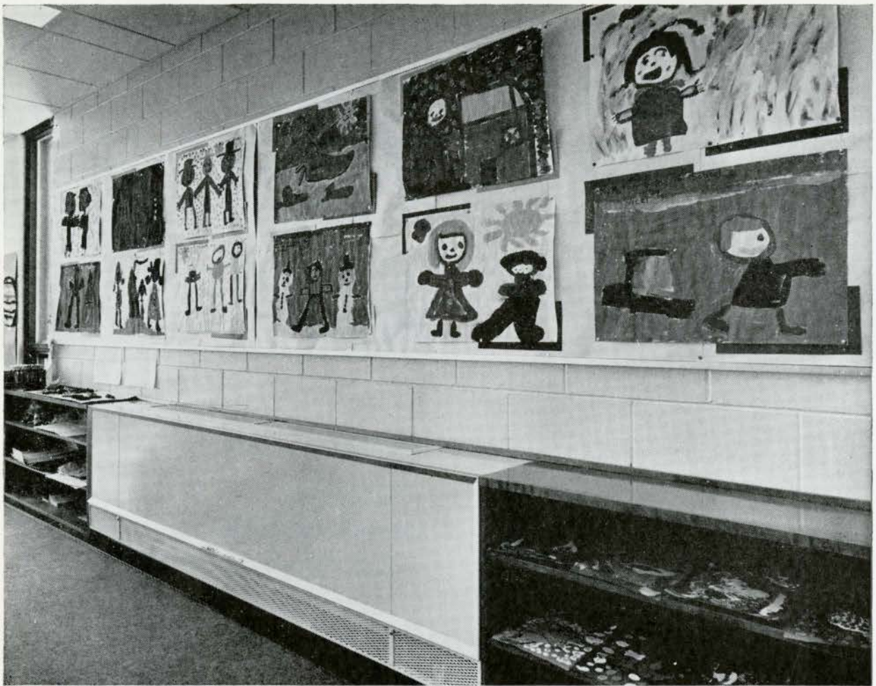
One of the electric unit ventilators at Redwood Public School. Consulting Engineer: Howard Boland, P.Eng. Architect: Jean-Paul St. Jacques, M.R.A.I.C.
