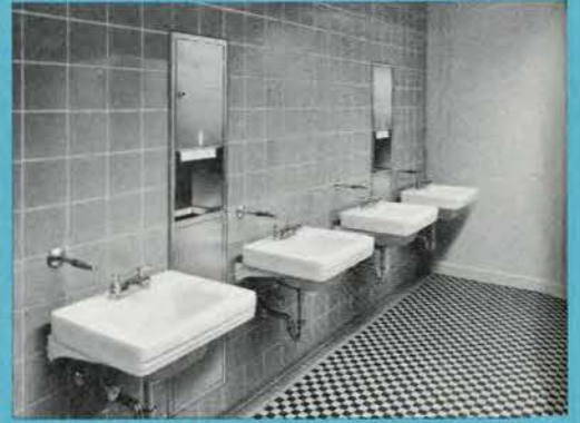
Typical Washroom Installation
