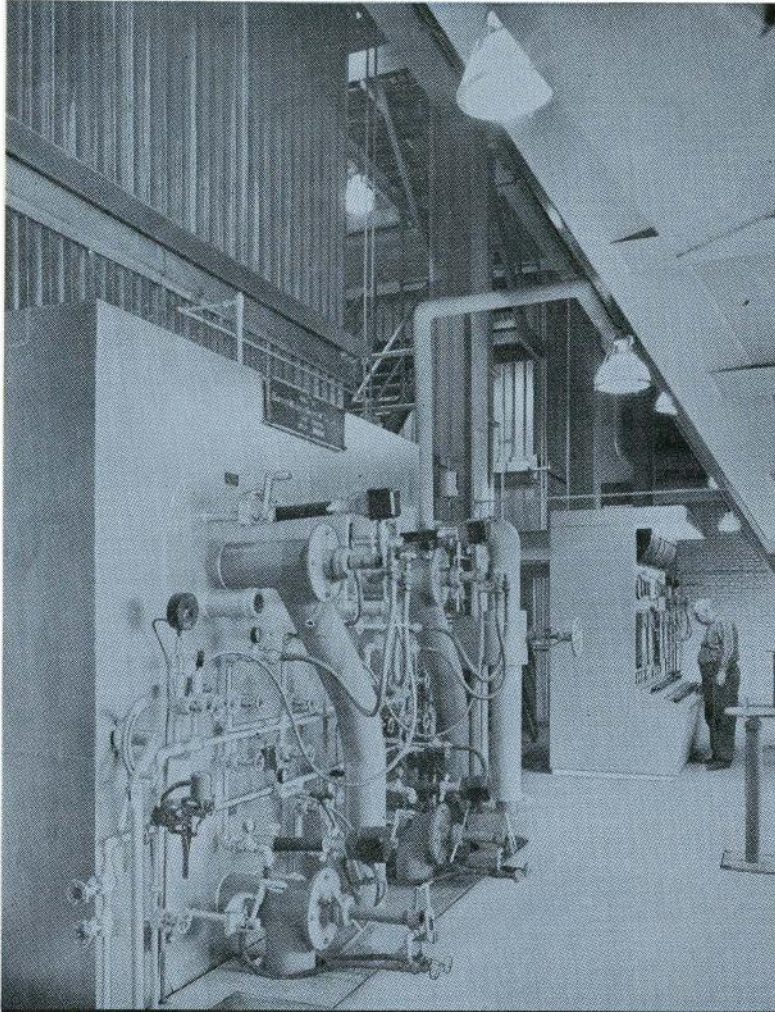
Two, 2-drum B&W Stirling Boilers, in service
