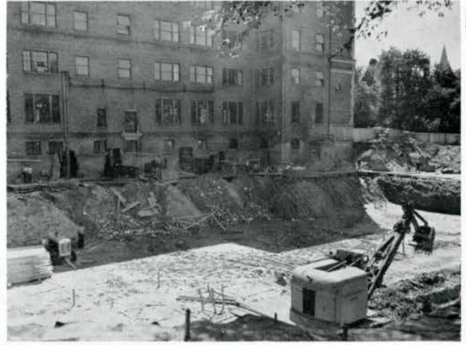
This illustration shows a general view of the underpinning operations on the north wall of the existing building. Note the beam left at the existing building.
