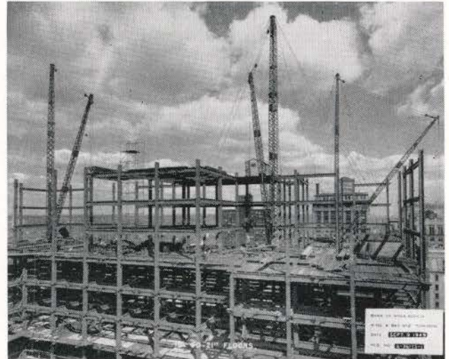
This illustration shows the commencement of steel erection between the 19th and 21st floors. A good view is obtained of the cantilever spandrel construction. K bracing can be seen at the extreme left. 9 September, 1949.
