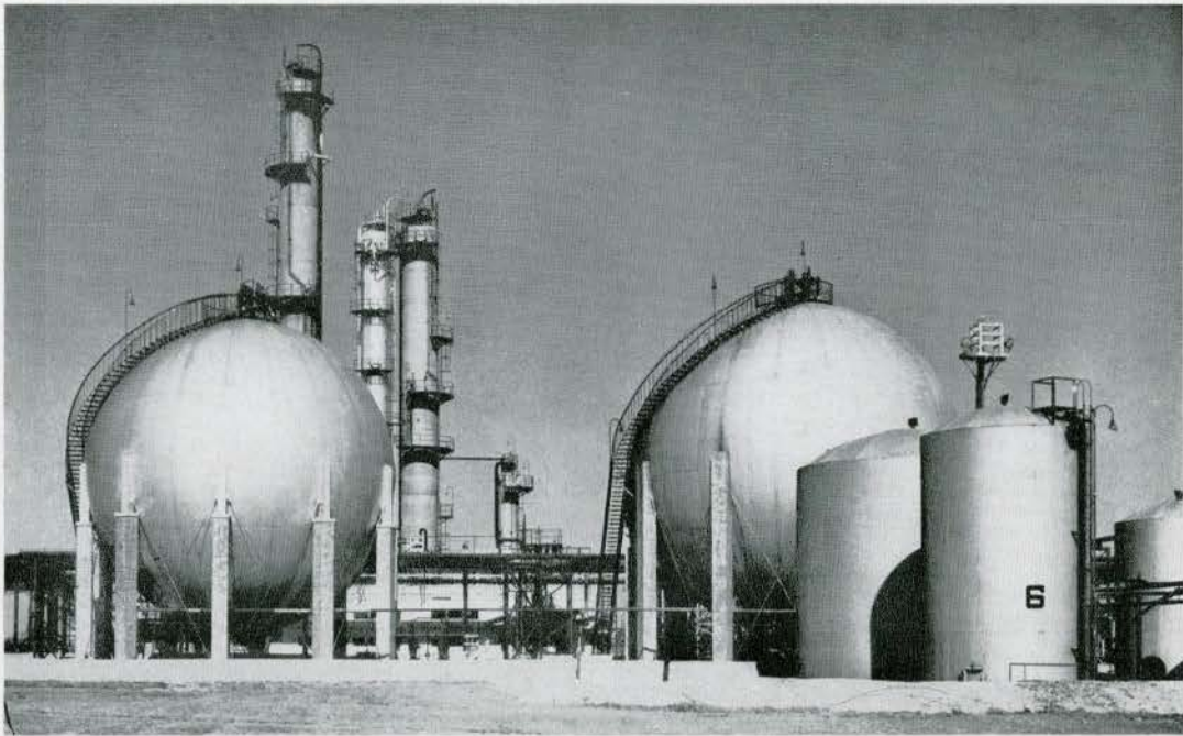
STORAGE TANKS IN FOREGROUND. BUTYLENE CONCENTRATION TOWERS IN BACKGROUND
