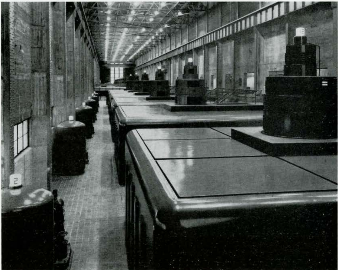
INTERIOR OF SHIPSHAW NO. 2 POWERHOUSE
