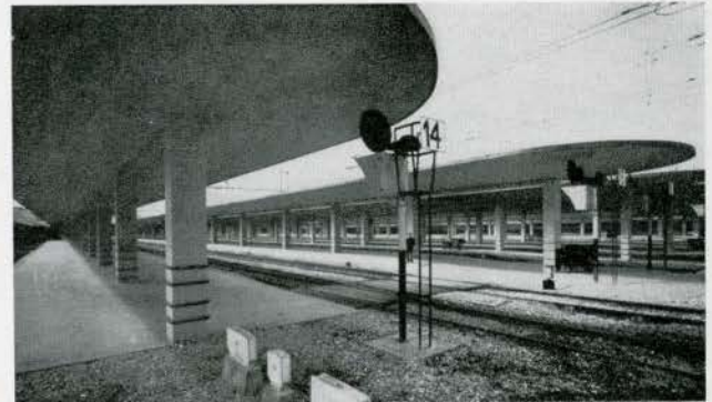
View of the platforms: The boldly cantilevered canopy is composed of reinforced concrete with a soffit of coloured marble mosaic.
