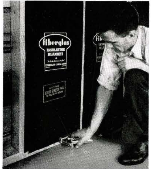
Roll Blankets are enclosed in vapor paper. The blanket is placed between the studs. Paper is tacked with lath nails.
