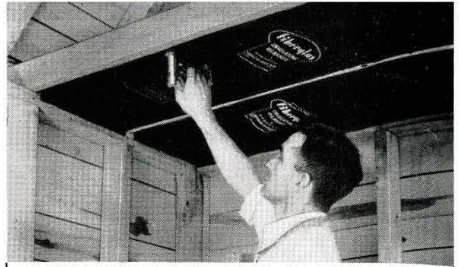
Fiberglas is installed in ceilings and roofs the same as in walls.
