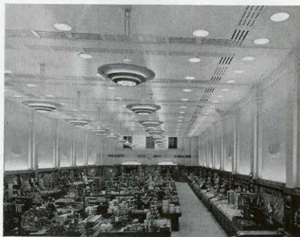
Photo (above) shows an unusual and decorative handling of inlets from conditioned air ducts which are insulated with corkboard.
