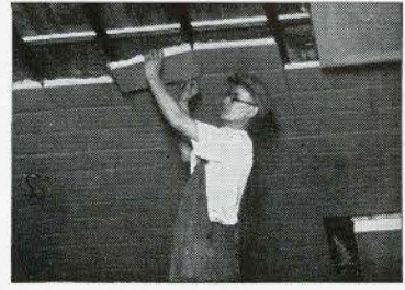
300,000 square feet of J-M Sanaoustic Tile applied in these offices reduced errors 42%—representing a return of 67% per year on the cost of installation.
