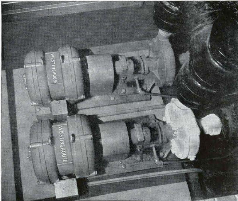
View from above of Westinghouse motors driving De Laval Brine Pump, furnished through Canadian Ice Machine Company. (Above)
