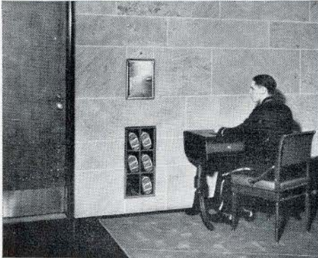
Air-tite Receiving and Dispatching Terminal set in marble wall on Melinda Street Mezzanine. Bull's eye signal light above door to announce arrival of a carrier. Carrier storage space below terminal door.
