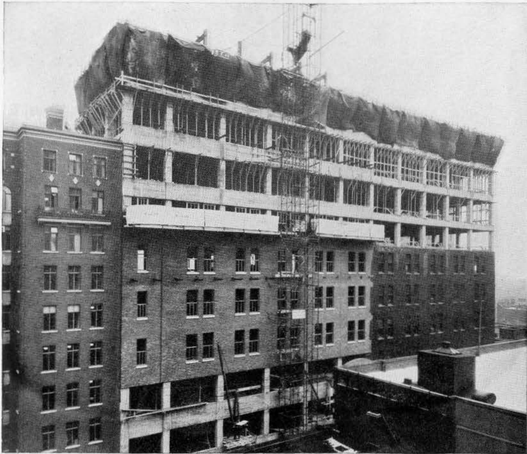
Progress picture of the extension to the Elgin Exchange, Bell Telephone Co., Toronto. Chapman and Oxley, Architects.
