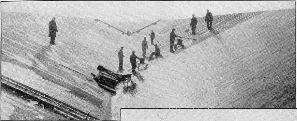
Above—Applying a Murray-Made 20 Year Bonded, Built-Up Asphalt Roof over saw-tooth roof of new foundry building of Robert Mitchell Company, Limited, at St. Laurent, P.Q. Architects, T. Pringle & Sons Ltd.; General Contractors, Anglin-Norcross Ltd.; Roofing Contractors, Geo. W. Reed & Co. Ltd.,—all of Montreal.
