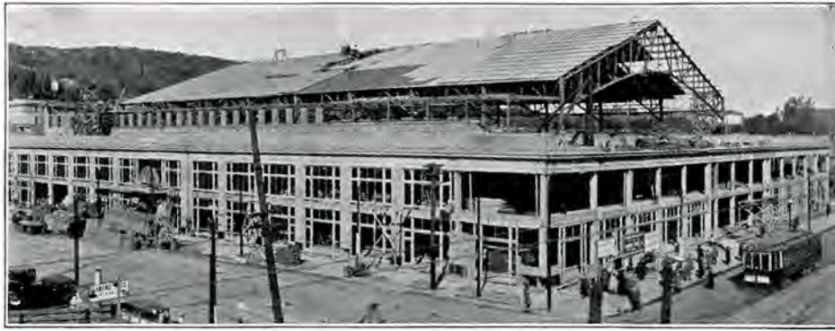
New Montreal Forum. Entire building, with exception of the roof, is of reinforced concrete construction. Seating capacity 9,000 to 13,000. Erected in less than four months. The Atlas Construction Company, Limited, were the contractors
