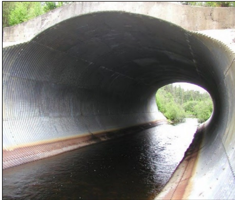
Figure 2.8 Invert corrosion of a CMP culvert (Hansen, 2007).
