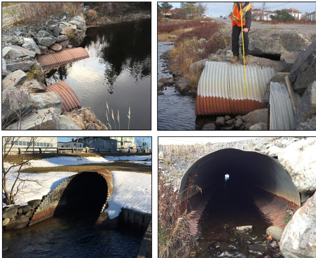
Figure 5.1 Examples of corroded CMP culverts in Canada (Campbell, 2017)
