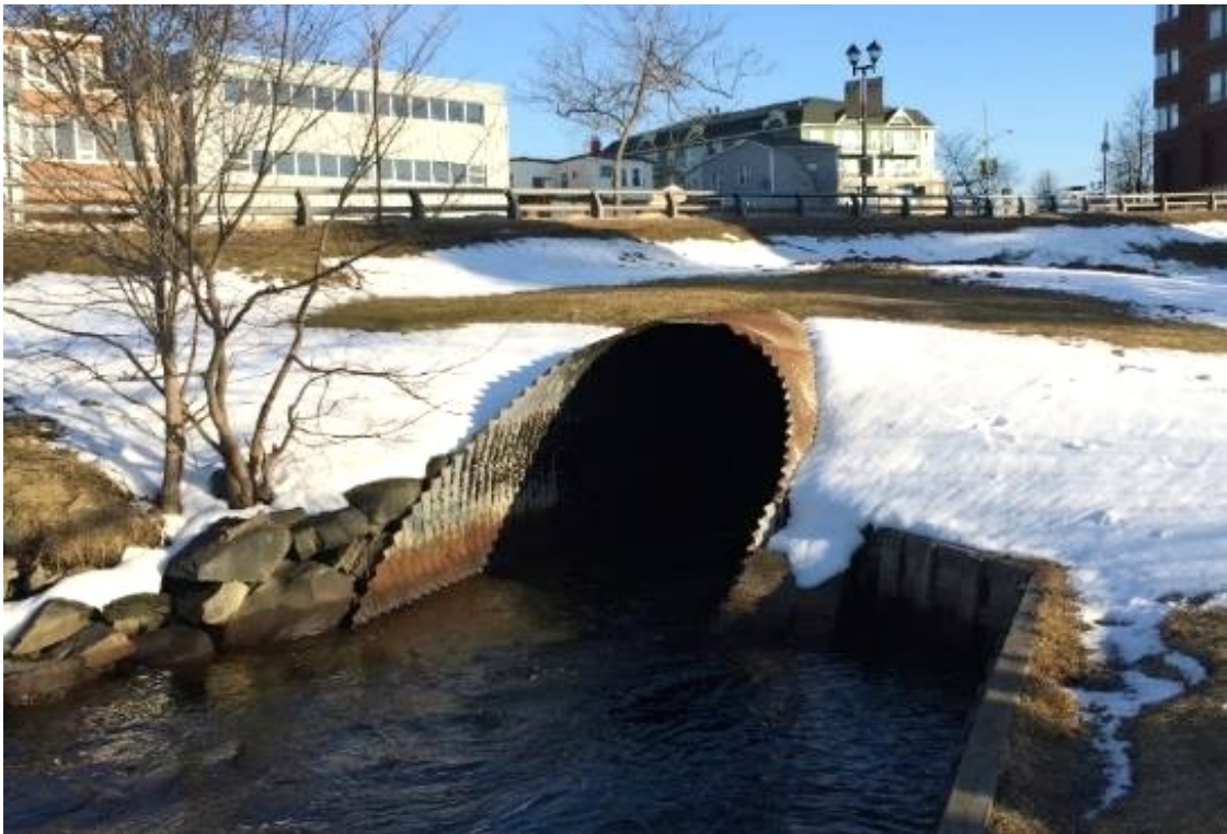
Figure 1.3 CMP culvert in Dartmouth, Nova Scotia exhibiting corrosion at the crown and haunches. (Campbell, 2017)
