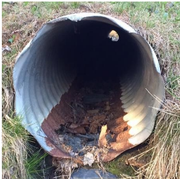
Figure 1.2 CMP culvert in Halifax, Nova Scotia exhibiting severe corrosion along the invert (Campbell, 2015)
