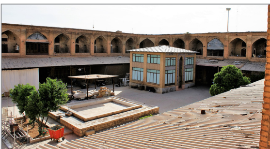
Figure 11: A deteriorating caravanserai adjacent to the bazaar
