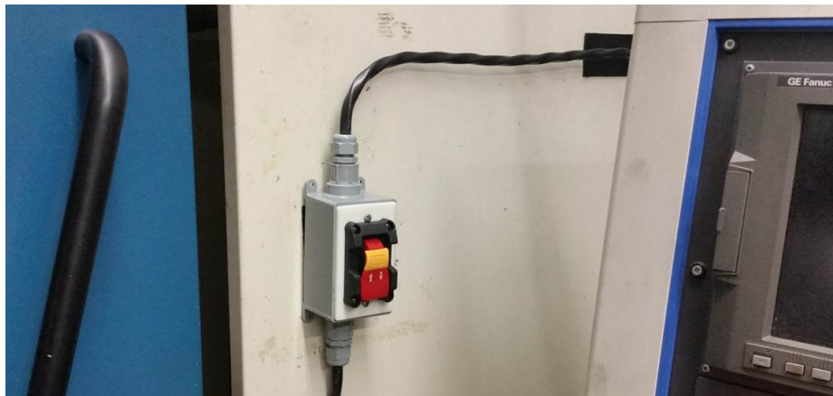
Figure 4.9: Emergency stop switch
