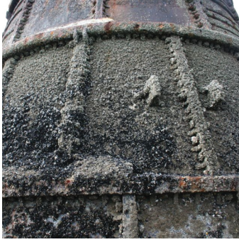
Figure 57 Detail image of the Whitford modular bolted plates rusting (Emmanuel, 1985)
