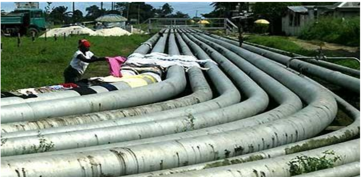
Figure 36. Criss-cross surface pipelines laid few meters from homes (Udo, 2014).
