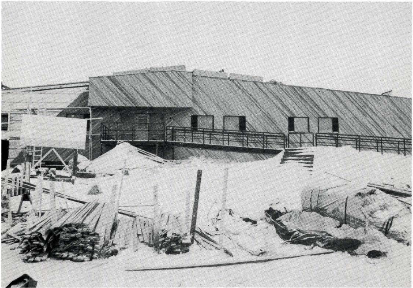
Pelly Bay school under construction throughout the winter of 86/87. Utmost simplicity was the key as it all came in the belly of a Herc.
