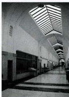
Fig. 8. Filter gallery looking towards the filter rotunda, with glazed screen to filter bed at left. (S. Mannell, 1998.)
