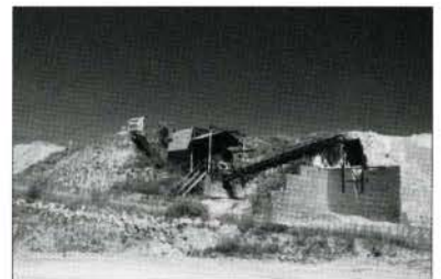
Fig. 31. Clay storage and mixing area on the edge of clay embankment, I-XL site. (E. Mills, August 1999)
