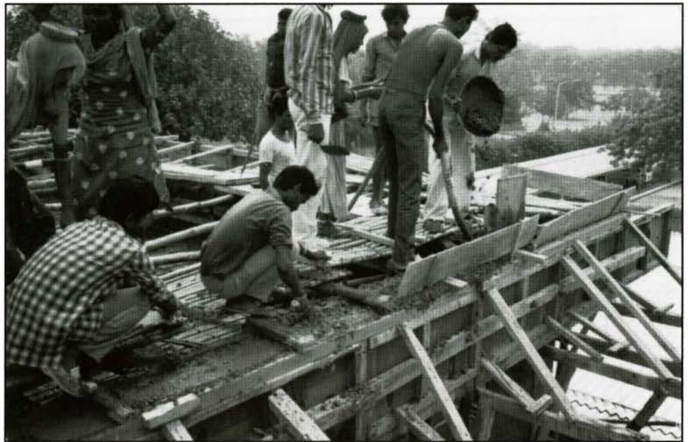
Fig. 4. Construction workers during the building of the second phase of the High Commission, c. 1990. Department of Foreign Affairs and International Trade (DFAIT)
