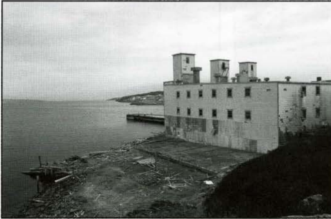
Fig. 37. Side elevation of fish plant with the foundations of the salt store on the left. (Photo: R. Goodspeed, 1998)
