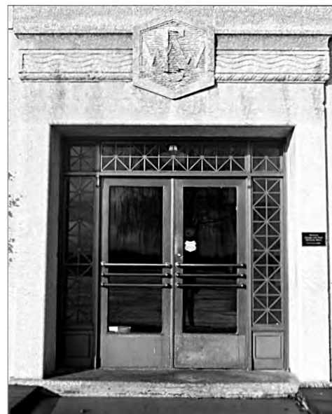
FIG. 14. GLENMORE WATER WORKS. DETAIL OF THE MAIN ENTRY DOOR SHOWING THE ORNAMENTAL BRONZE WORK, AND THE WAVE-FORM FRIEZE BRACKETING THE HEXAGONAL MEDALLION CARVED WITH THE "CWW" MONOGRAM. | STEVEN MANNELL, 2001.
