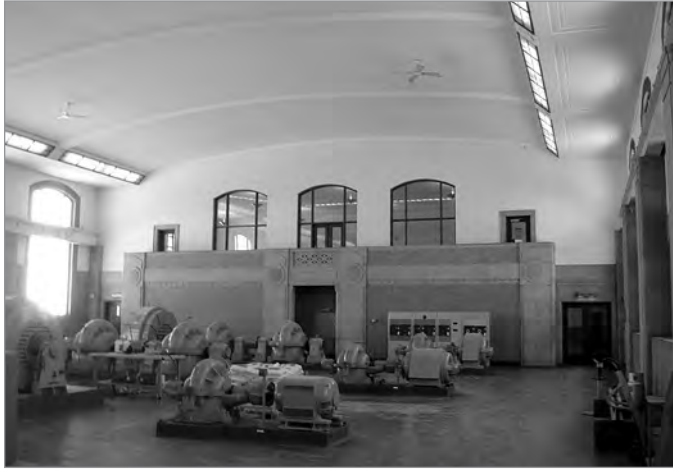
FIG. 2. INTERIOR VIEW OF THE PUMPING STATION, VICTORIA PARK WATER WORKS, SHOWING THE VAULTED PLASTER CEILING AND COVE LIGHTING AT THE EAVES, ALONG WITH THE TILE FLOORS, TILE WAINSCOTING TRIMMED WITH QUEENSTON LIMESTONE, AND THE VIEWING BALCONY IN FRONT OF GLAZED SCREENS GIVING ON TO THE PUMPING CONTROL ROOM. THE SUSPENDED PLASTER CEILING IS UNIQUE AMONG WATERWORKS PUMPING STATIONS. | STEVEN MANNELL, 2008.
