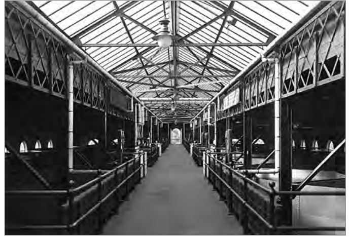
FIG. 8. VIEW OF THE FILTER GALLERY OF THE DRIFTING-SAND FILTRATION PLANT AT CENTRE ISLAND, AUGUST 27, 1918. THE CENTRAL SKYLIT ACCESS PLATFORM IS FLANKED BY RANKS OF CYLINDRICAL RIVETED STEEL GORE-RANSOME FILTERS; THE PLATFORM WIDENS TO HOUSE THE FILTER OPERATING CONTROLS. THE STRUCTURE IS LEFT ENTIRELY EXPOSED, WITH NO DECORATIVE FINISHES OR MATERIALS. | ARTHUR GOSS. CTA, SERIES 372, SUBSERIES 72, ITEM 896.
