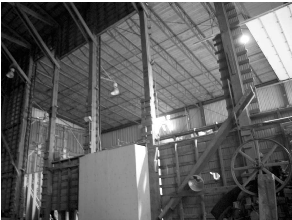
Snyder's main building - note holes cut into walls
