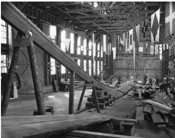
Bluenose II keel laid in shed - note diagonal lateral bracing (Government of Nova Scotia, n.d.)
