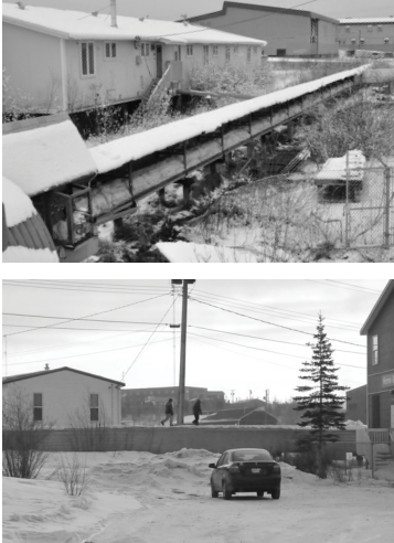
Figure 57: Above grade utilidor for basic services in Inuvik, Canada; from Morin, “Life in Inuvik, Northwestern Territories”
