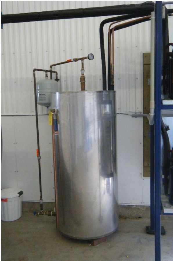
Figure 4: A heat recovery unit installed in one of the audited dairy farms
