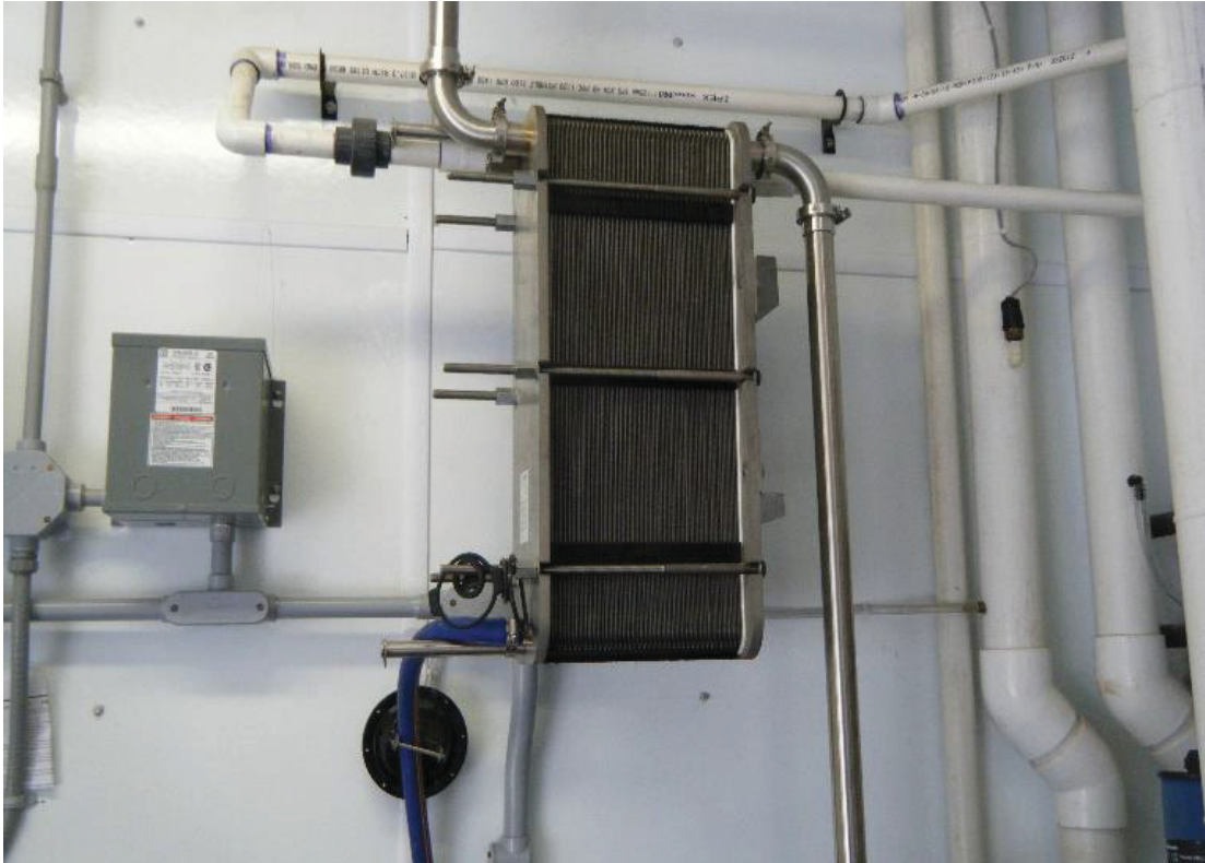
Figure 2: A pre-cooler installed in one of the audited dairy farm to cool milk from the cow
