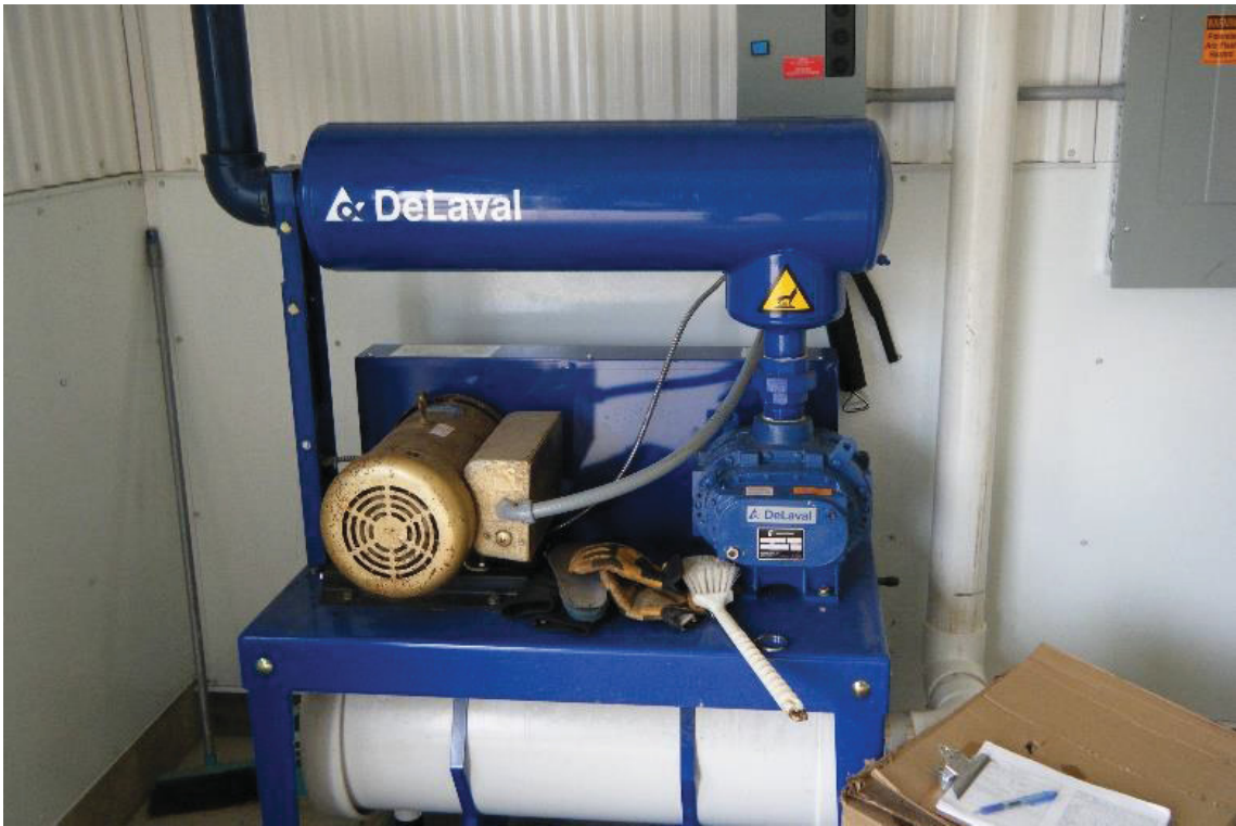
Figure 5: Vacuum pump and motor
