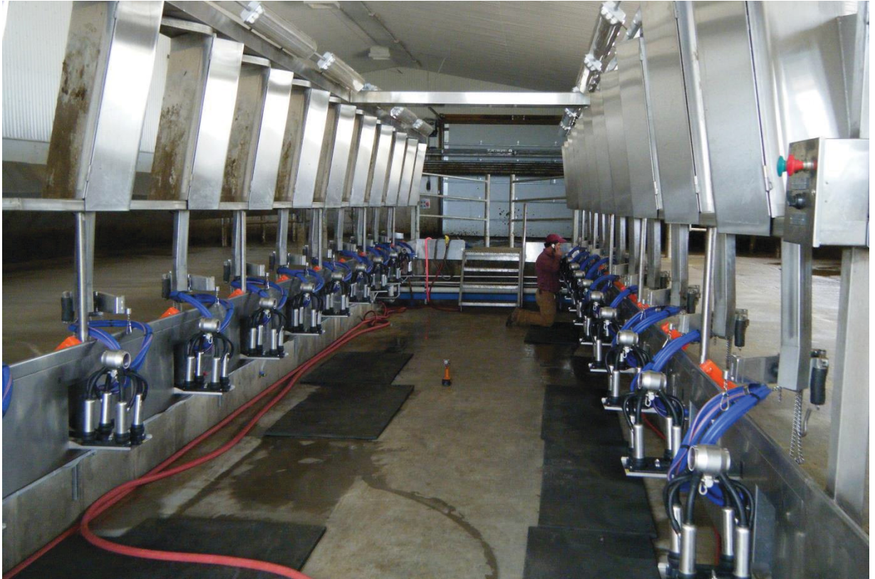
Figure 7: T8 lights installed in milking parlour
