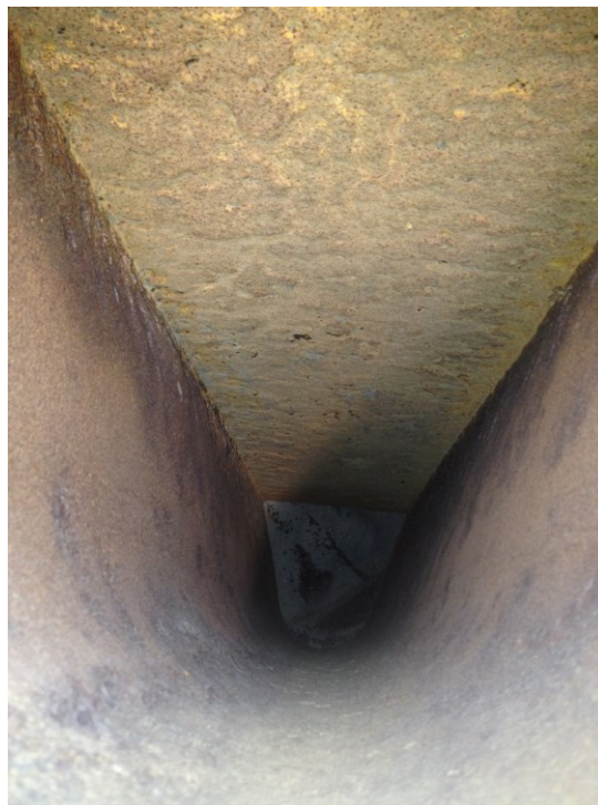
Figure D.34: Specimen C5 inside of stiffening rib.
