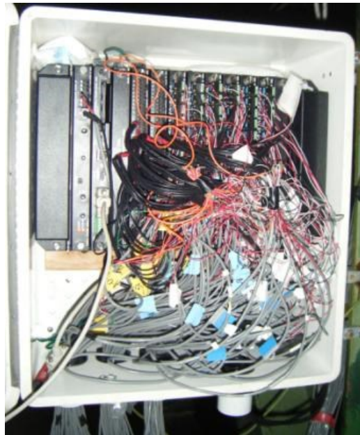
Figure A.8: Datalogger completed wiring.
