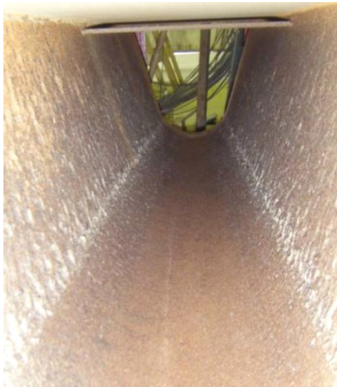
Figure 7.27: Inside rib plate, specimen C10.
