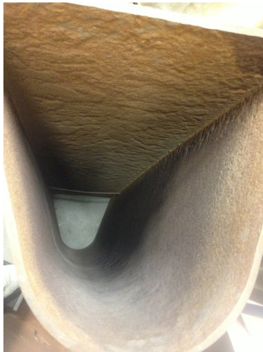
Figure D.32: Specimen C4 inside of stiffening rib.
