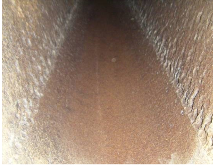
Figure D.31: Specimen C10 bottom of stiffening rib.
