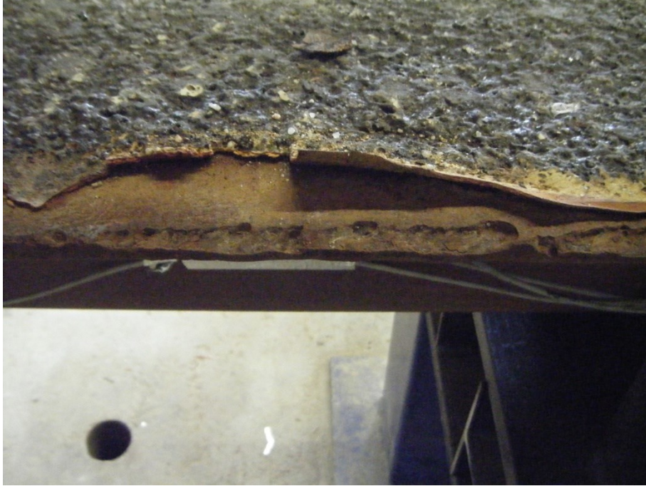
Figure D.41: Specimen C2 corrosion on deck along length of specimen.
