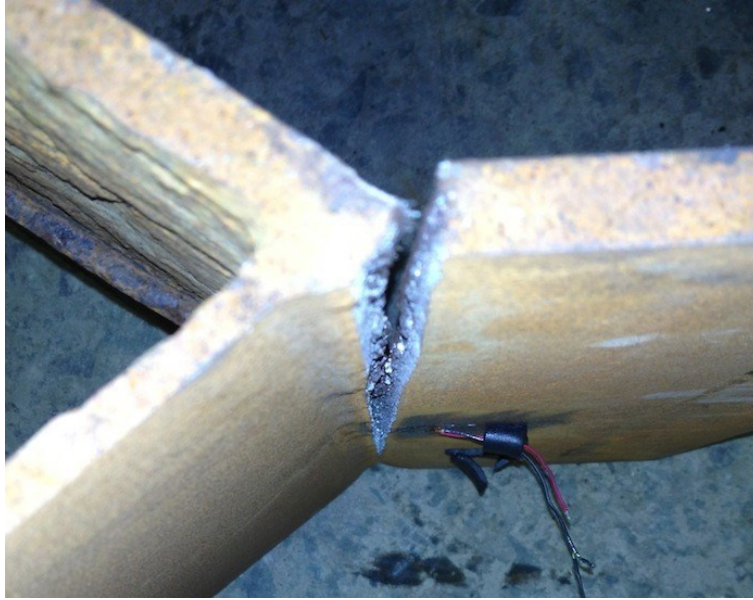
Figure 7.10: Toe-deck cracking on specimen A5.
