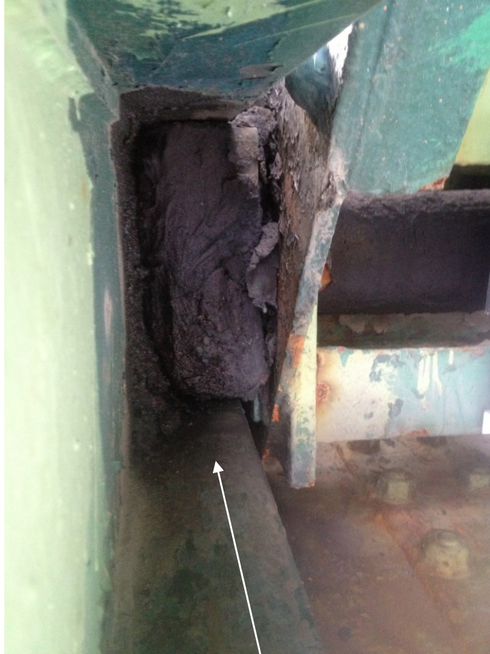
Figure 3.10: Sliding bearing at DMT MS, South side
