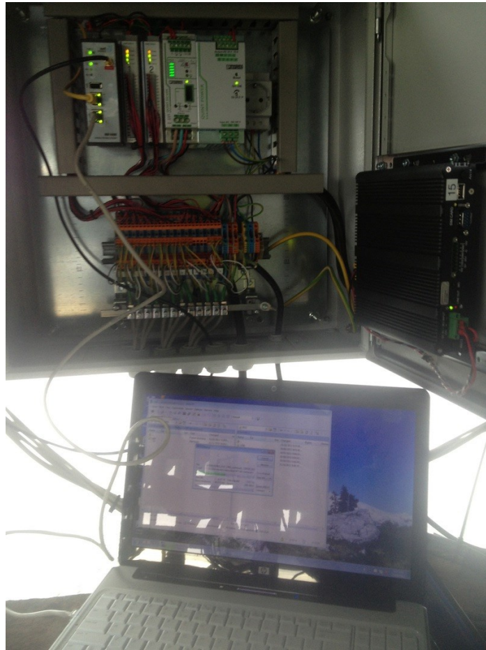
Figure 5.5: Monitoring box and field laptop for manual download
