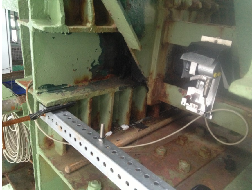
Figure 5.2: Typical bottom wire displacement sensor mounted to bearing crosshead
