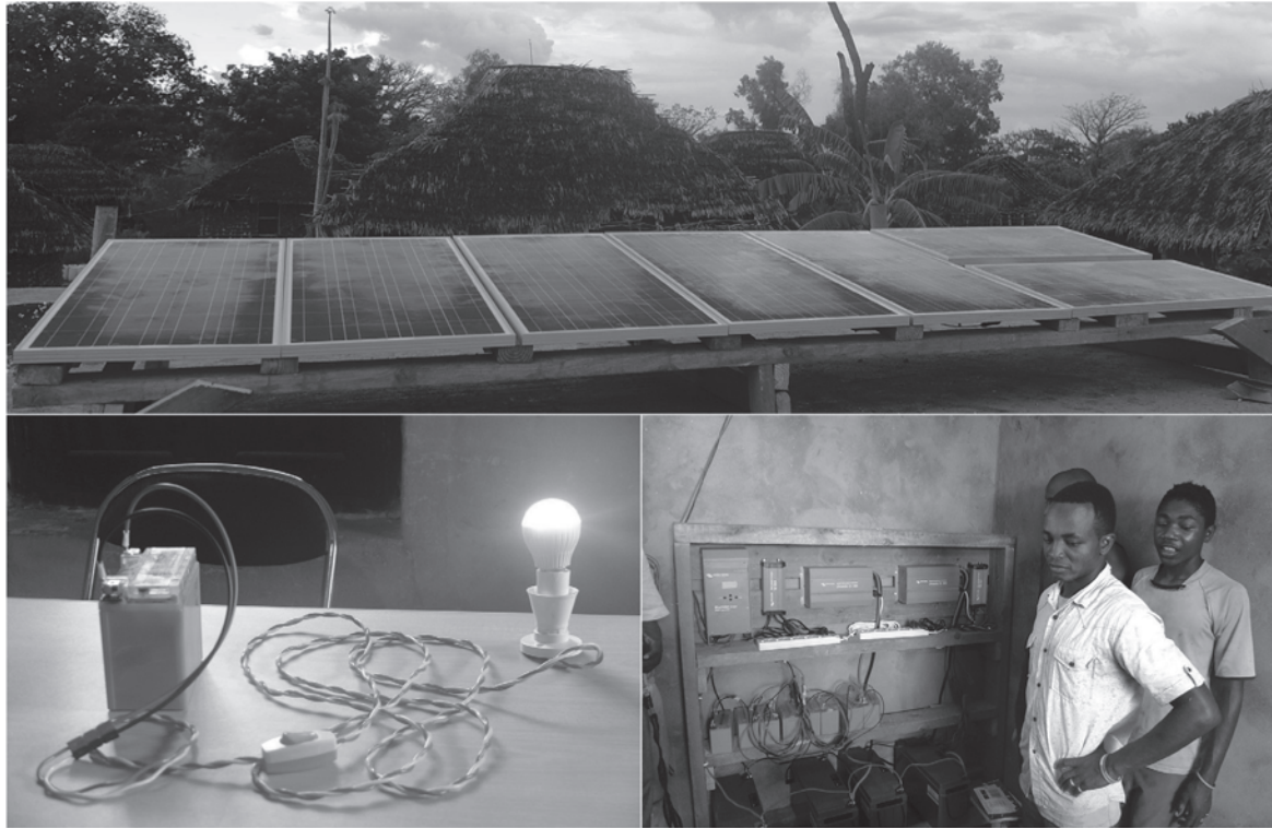
PV installed in Kokota (top), a household lighting system (bottom left), and Kokotans waiting for their batteries to charge (bottom right).
