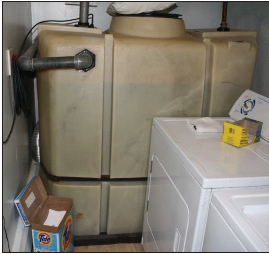
Figure 4.3 Potable water storage tank inside house, approximate capacity of 1200 litres (photo credit: first author)
