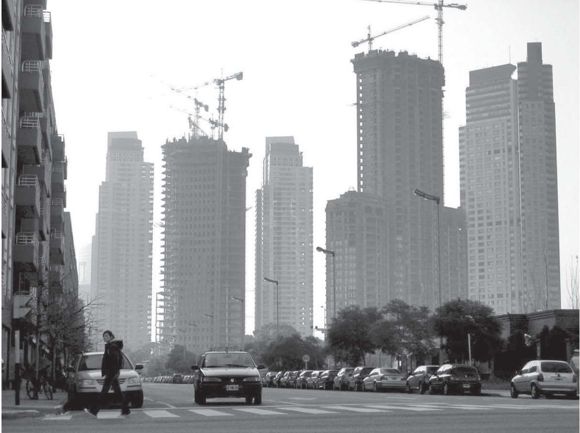
Buildings under construction in the formal city of Buenos Aires (Skyscraper City 2008)
